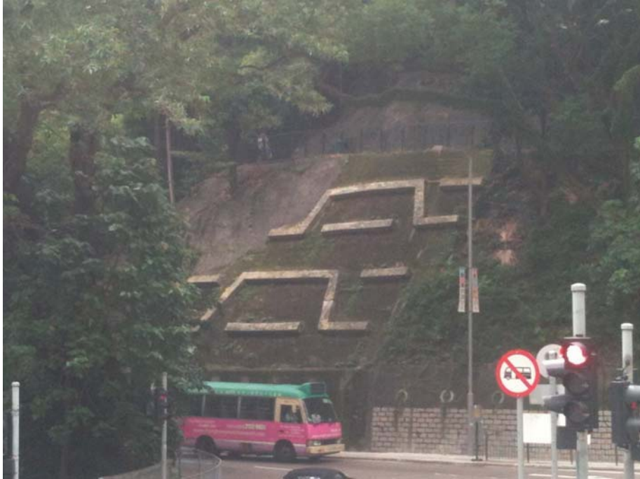
Photo 17 : Profiled finishes on the external faces of slopes to be avoided
