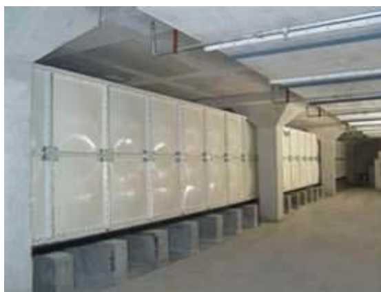
Photo 23 : Glass Reinforced Water Tank
