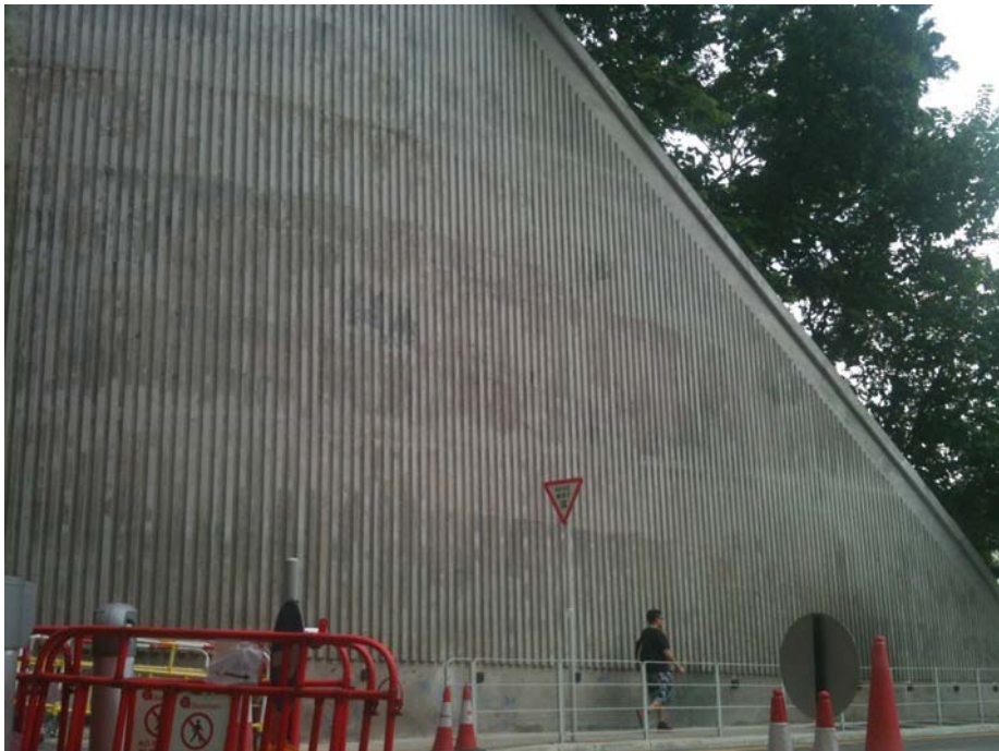
Photo 18 : Profiled finishes on the external faces of retaining walls to be avoided
