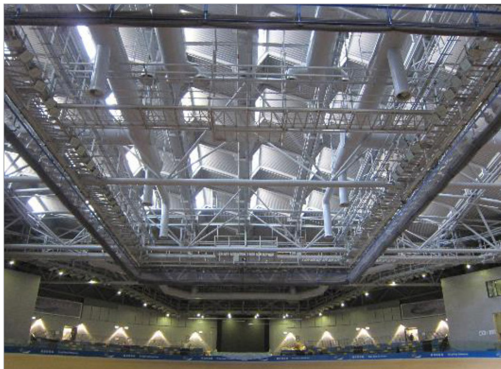
Figure 5 Overview of the cat walk system
