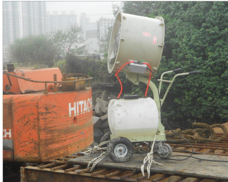
Figure 5 The deodorizing unit for dredging operation
