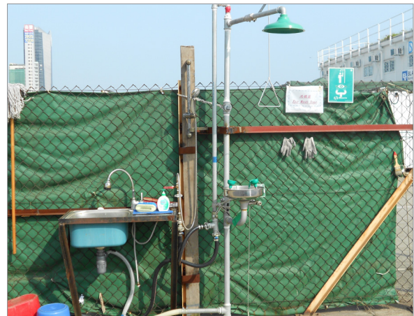
Figure 9 Emergency washing facilities
