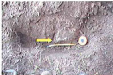
Large Root Severed (arrow). Smaller, cut roots can be seen throughout excavation
