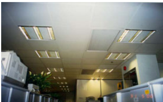
Fig. 10 Lighting after retrofit with new T5 luminaires
