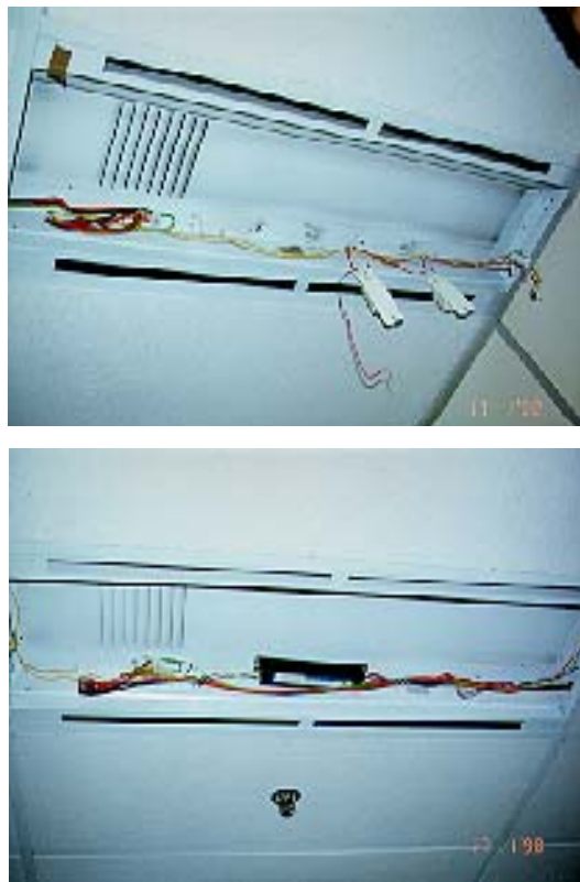
Fig. 5 Replacement of 2 nos. 36W Conventional Ballasts by 1 no. Electronic Ballast in Luminaire at Harbour Building
