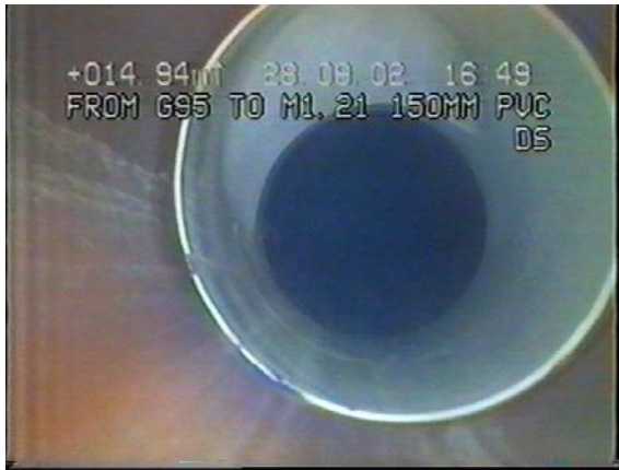
Plate F19 Pipe Material Change
