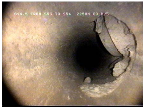
Plate F10 Connection Defect with Intruding Pipe
