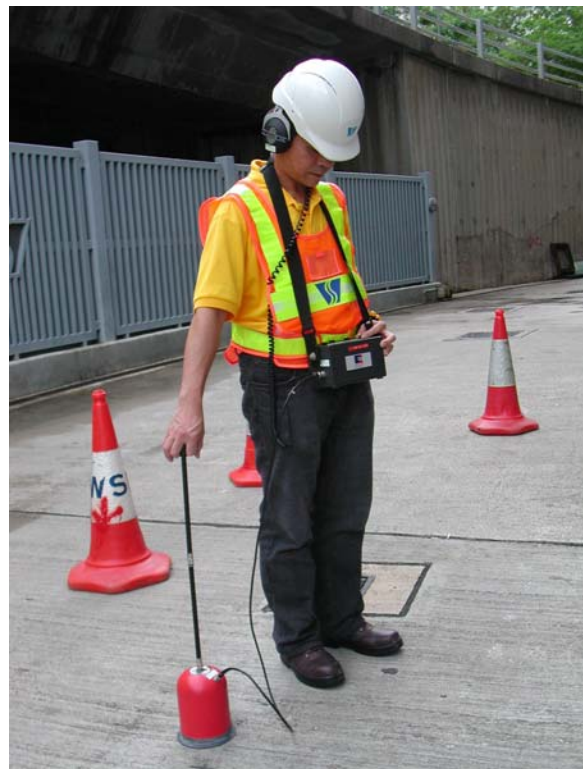
Plate H4 Leak Pinpointing by ELD
