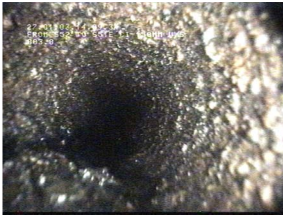
Plate F15 Heavy Scale on Pipe Wall
