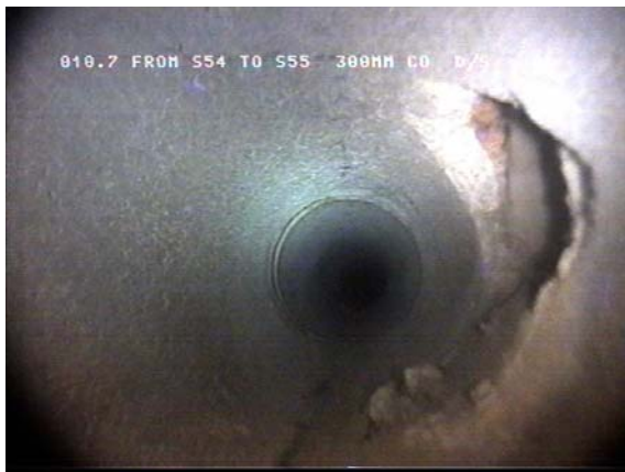
Plate F9 Connection Defect in Pipe
