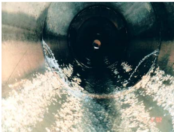
Plate F3 Water Infiltration into Pipe
