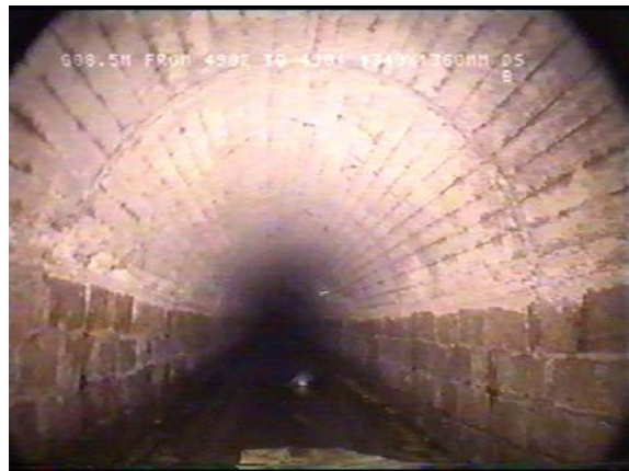
Plate F8 Spalling of Pipe Wall
