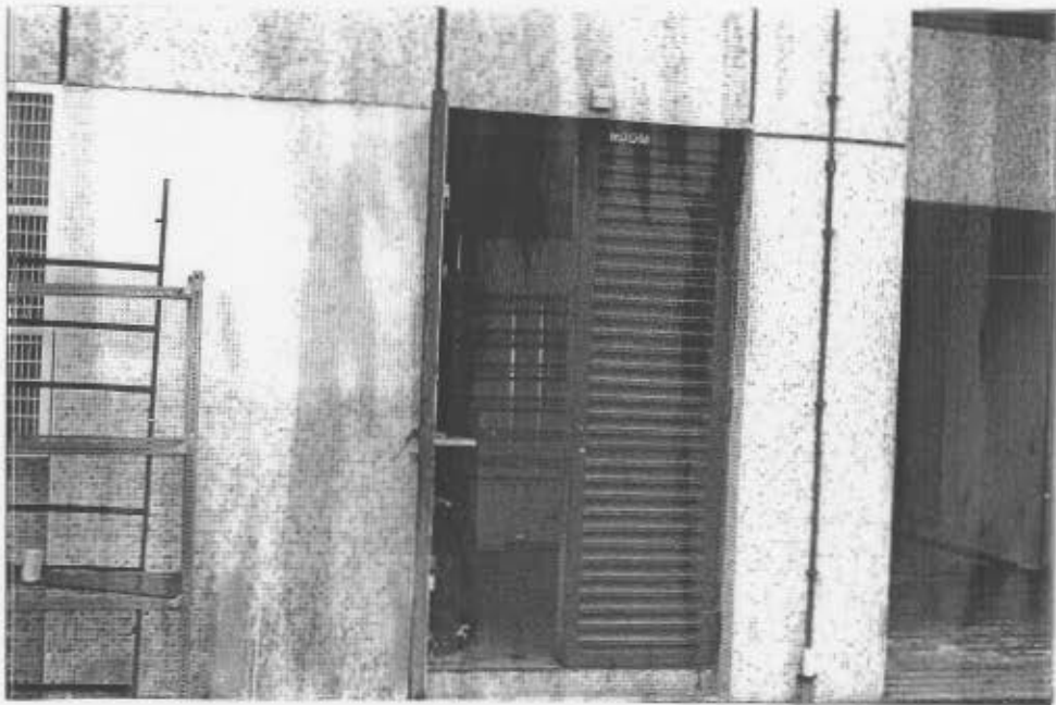
Plate 2 - Storage Room at Ground Floor Level of the Public Works Central Laboratory Building
