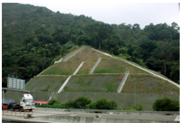
Plate 2 - Appearance of a cut slope along Tai Po Road before and after LPM works
