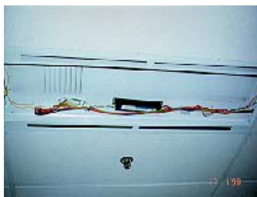
Fig. 5 Replacement of 2 nos. 36W Conventional Ballasts by 1 no. Electronic Ballast in Luminaire at Harbour Building
