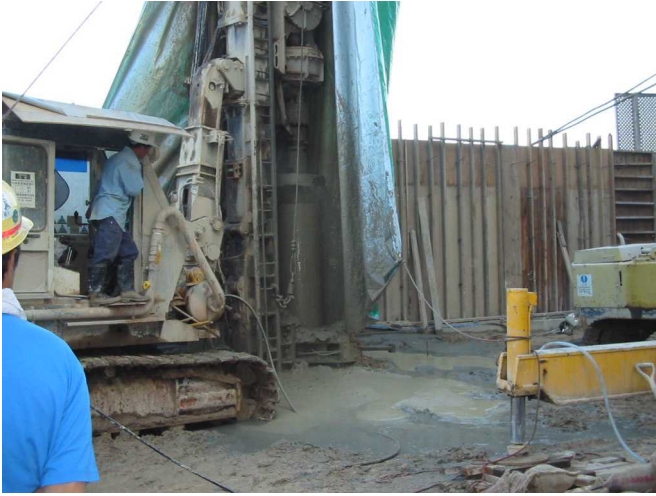
Photo 3: Drilling of piles for the Electrochlorination House near the seawall of the existing Tai Wan Salt Water Pumping Station
