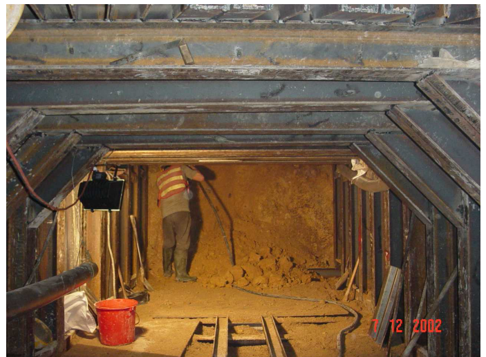
Photo 5: Manual tunnel excavation for installing the 1,000 mm fresh watermain and 800 mm salt watermain under Tsz Wan Shan Road at its junction with Po Kong Village Road
