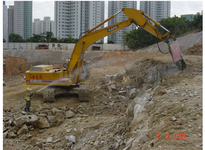
Photo 2: Rock Excavation to form platform at 74 mPD for Diamond Hill No2 Fresh Water Service Reservoir
