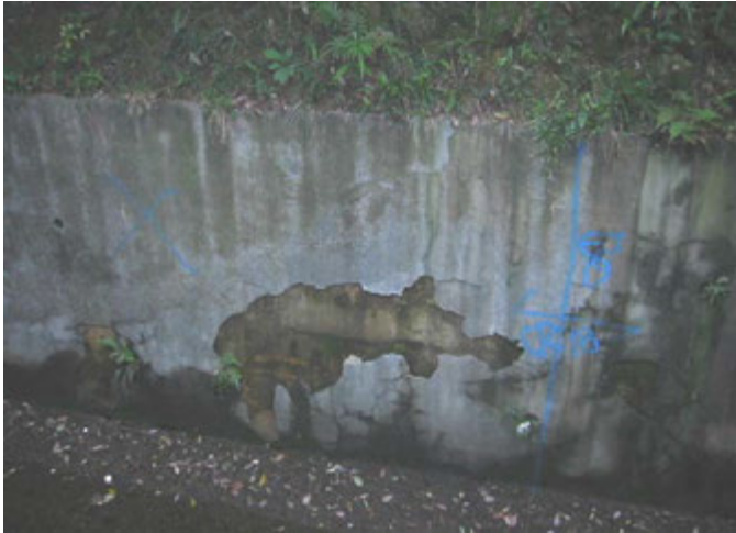
Figure 1 : Deteriorated condition of existing catchwater channel
