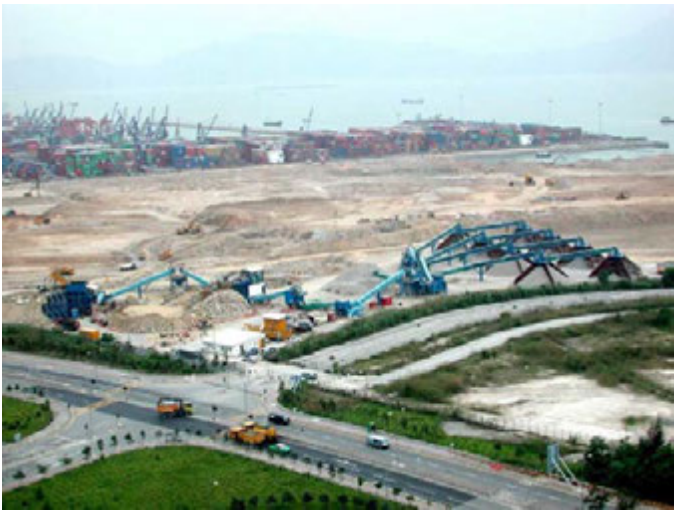
Figure 3 – Panoramic view of C&D material recycling facility at Tuen Mun Area 38
