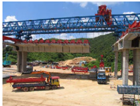
Precast segments are hoisted by the launching gantry 吊樑機將大型組件吊起
