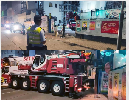
Temporary traffic arrangement to facilitate entry of heavy vehicles and material delivery from congested Jaffe Road
