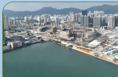
Completion of temporary reclamation of CKR (conceptual diagram for reference only): All temporary structures will be removed completely and the seabed will be reinstated
