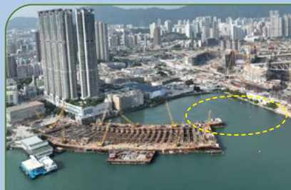
Temporary reclamation of CKR - Phase 2 (November 2022): Temporary structures from Phase 1 (i.e. circled on the right) have been removed and the seabed reinstated
