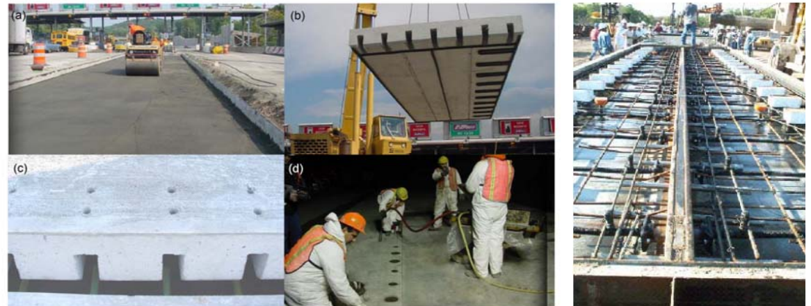
Complicate Joint Design: dowel bar + dent grouting (left); pre-stressing the joint (right)
