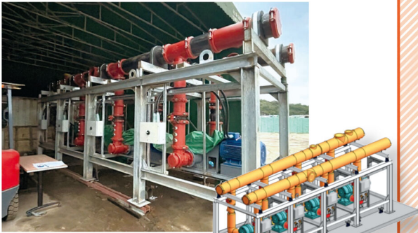
C 預製冷設備水泵 裝置模組裝嵌 Chiller Plant Pump Set Modular assembly
