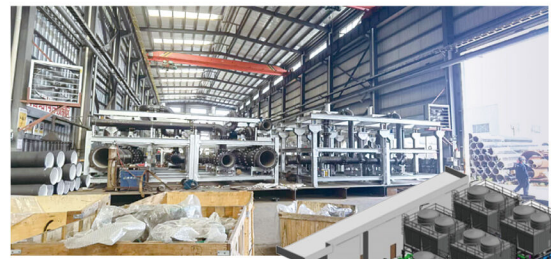
B 預製冷卻塔裝置模組 Pre-fabricated Cooling Tower Plant Module
