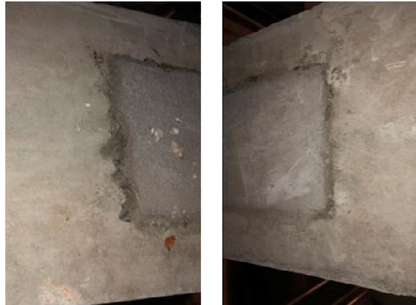
Bottom Face (No debonding found at the concrete/mortar interface)
