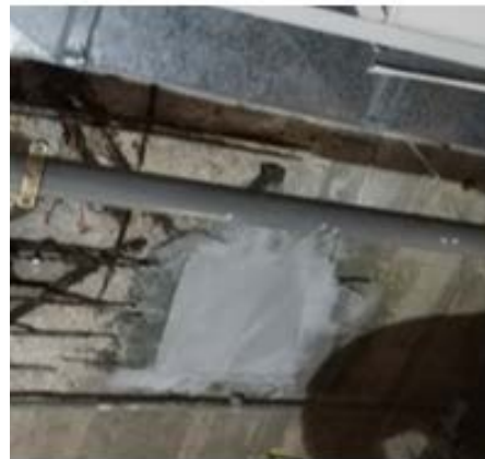
Ceiling at toilet
