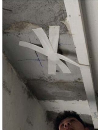
A suitable metal plate was glued to the cored hole and was pulled using a calibrated device until failure occurs.
