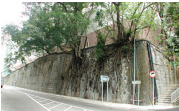
Plate 4 - Appearance of a retaining wall in the Mid-levels before and after LPM works
