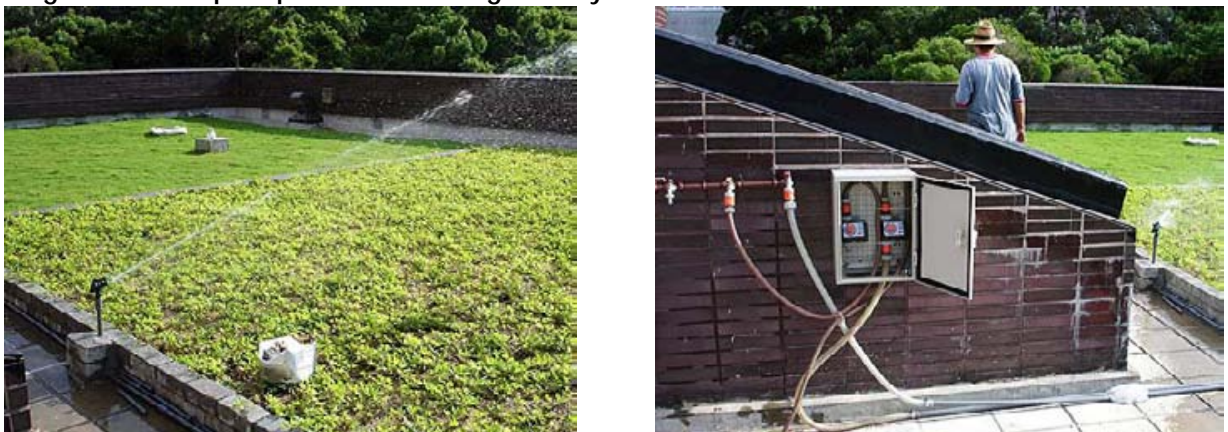
Figure 5.11 Simple Sprinkler Head Irrigation System
