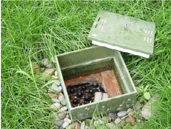
Inspection chamber for regular checking of the drainage layer. Drainage gullies should always have inspection chambers above. (Source and copyright © Greenlink Küsters Ltd.)
