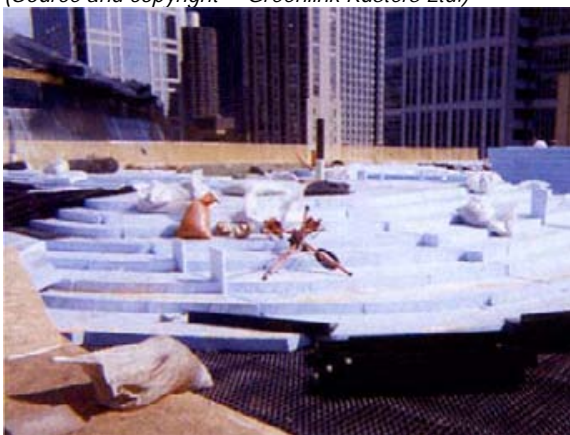
Light weight fills or additional thermal insulation layers are usually installed below the drainage layer. (Source and copyright © Earth Pledge, 2005)
