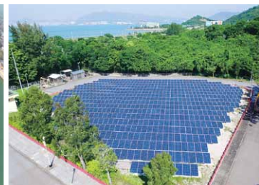
Photovoltaic System at Siu Ho Wan Sewage Treatment Works
